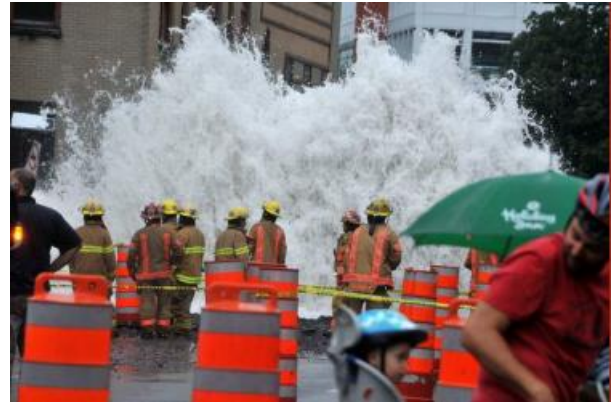
Figure 1: Example of a Montreal water main severed by a contractor during ground disturbance activities
